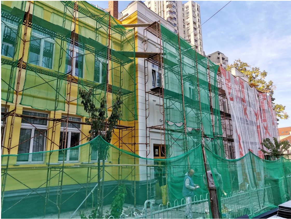
Pilot energy refurbishment of elementary school in Užice, Serbia, Photo: ©RDA Zlatibor
