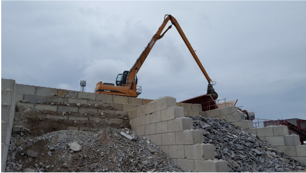
Fig. 14. Separate storage of delivered building rubble concrete and brick rubble in a recycling company and material removal by excavator
