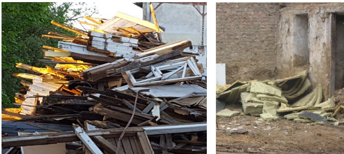
Fig. 12. Separated window frames (left), separated rock wool (right)
