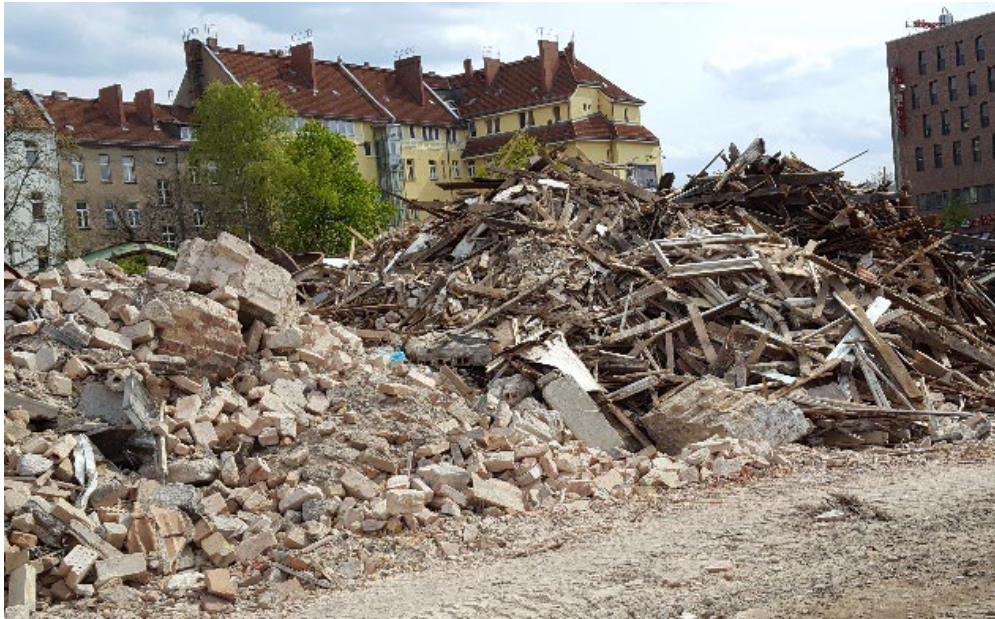
Fig. 11. Separation of brick from wood
