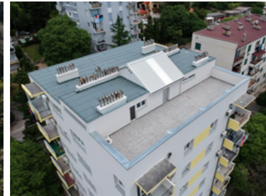
Drage Gervaisa 24, Rijeka – roof during reconstruction (resource: The Environmental Protection and Energy Efficiency Fund)
