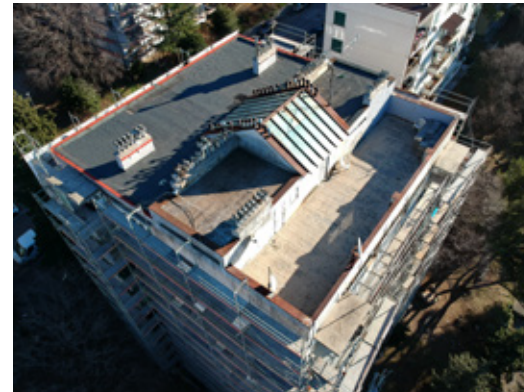
Drage Gervaisa 24, Rijeka – a roof before reconstruction (resource: The Environmental Protection and Energy Efficiency Fund)
